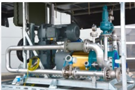
With flow meter
